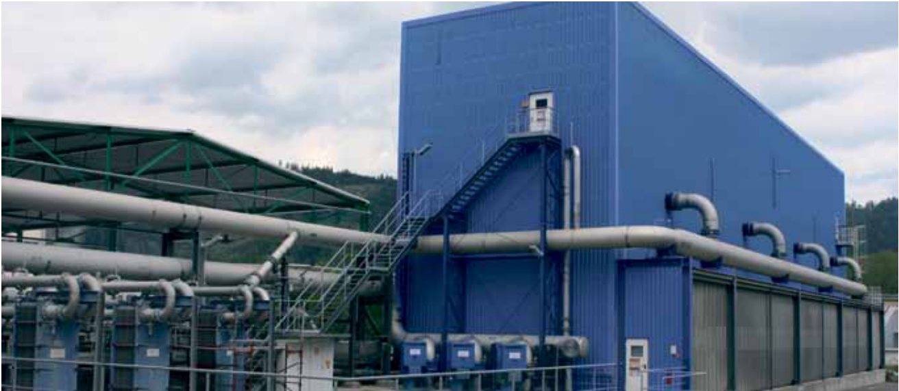
Figure 2: View on the four EWZ units of the cooling tower plant.
