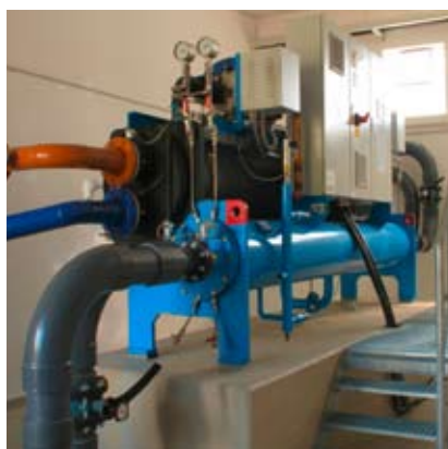
Heat pump in the machinery room of the outdoor swimming pool in Krumbach
